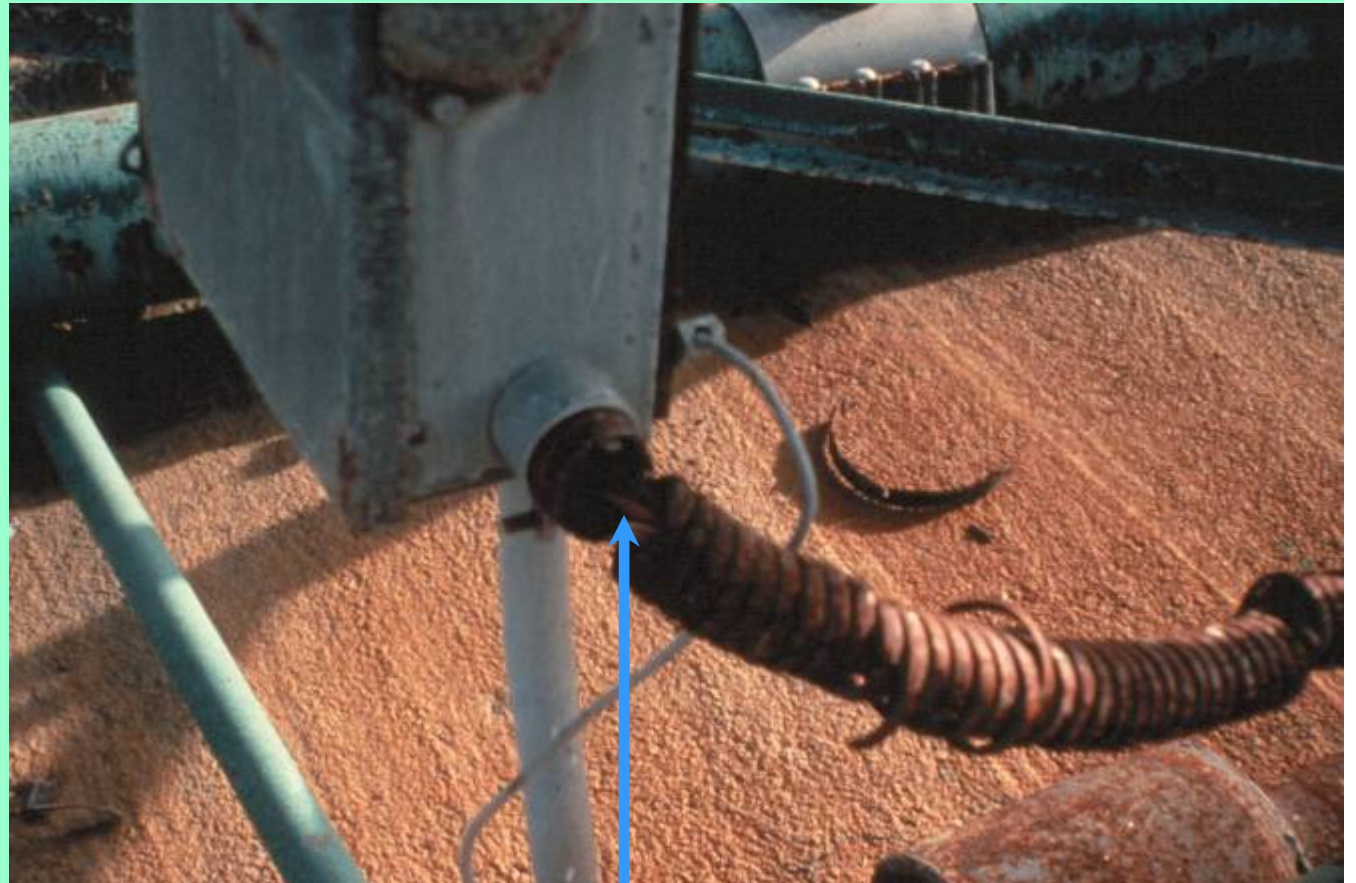
Old Corroded & Broken Conduit
