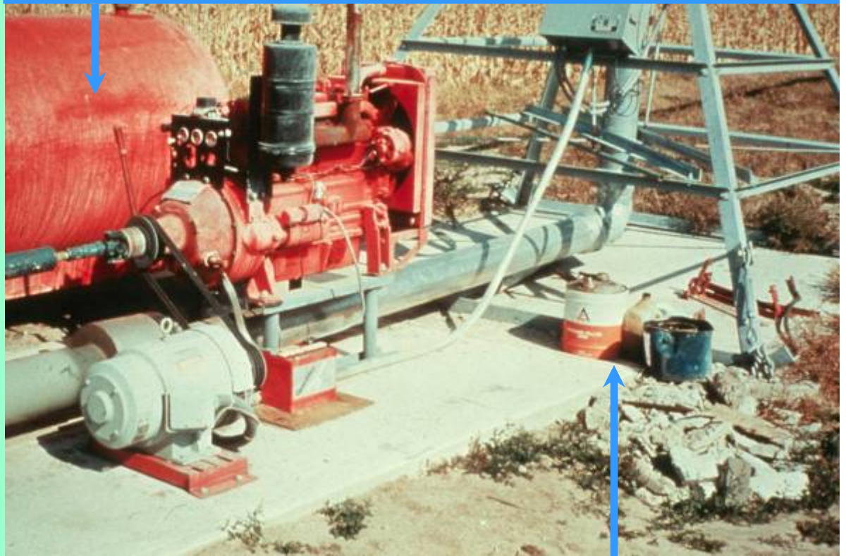
Fuel Storage Tank
